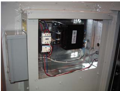
FIGURE 2: Electrical connection and high voltage disconnect.
